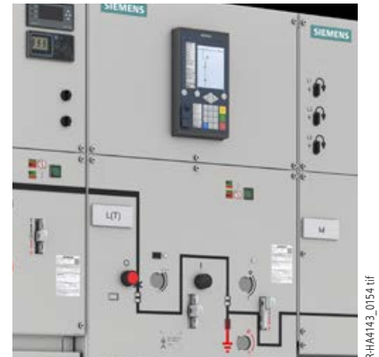
In circuit-breaker panel type L1(T) (750 mm)
